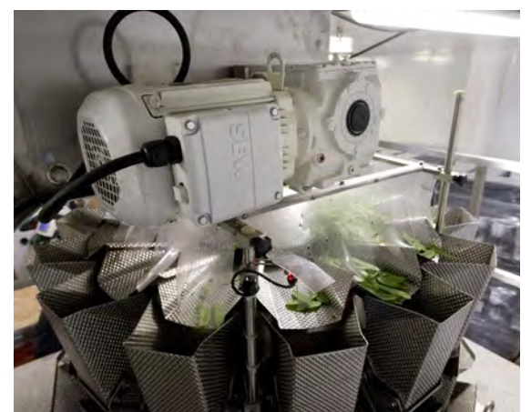
An SEW-Eurodrive motor provides smooth power distribution to the Bercy plant’s weigh scales.
